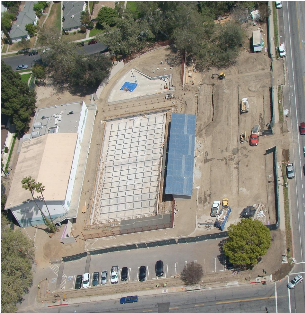
Verdugo Park Aquatic Facility looking east Mechanical building to right Bathhouse underneath recreation center on left
