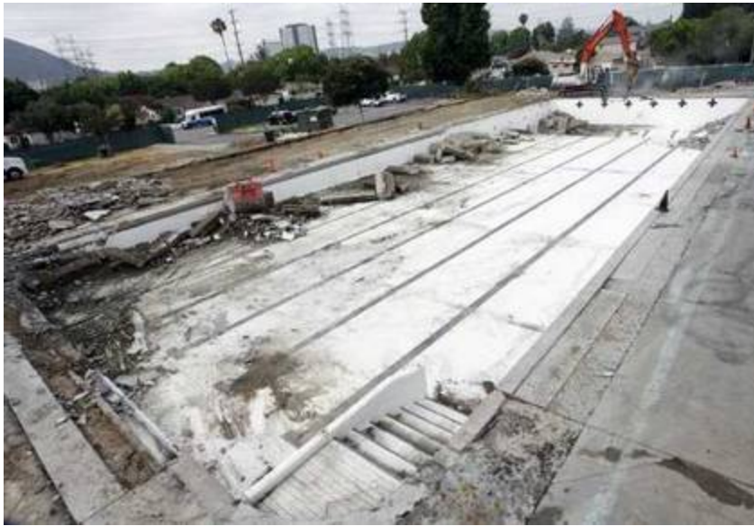
Construction workers remove the patio area around the Verdugo Recreation Center pool on Monday, July 16, 2012. (Times Community News / August 1, 2012)
